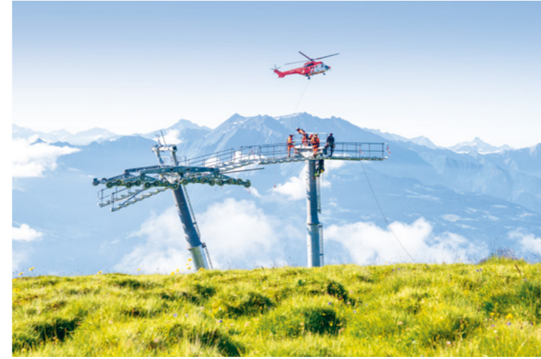
Tower Construction of Station Segnes – Nagens | FlemXpress | Flims | Switzerland Photo: © Philipp Ruggli
