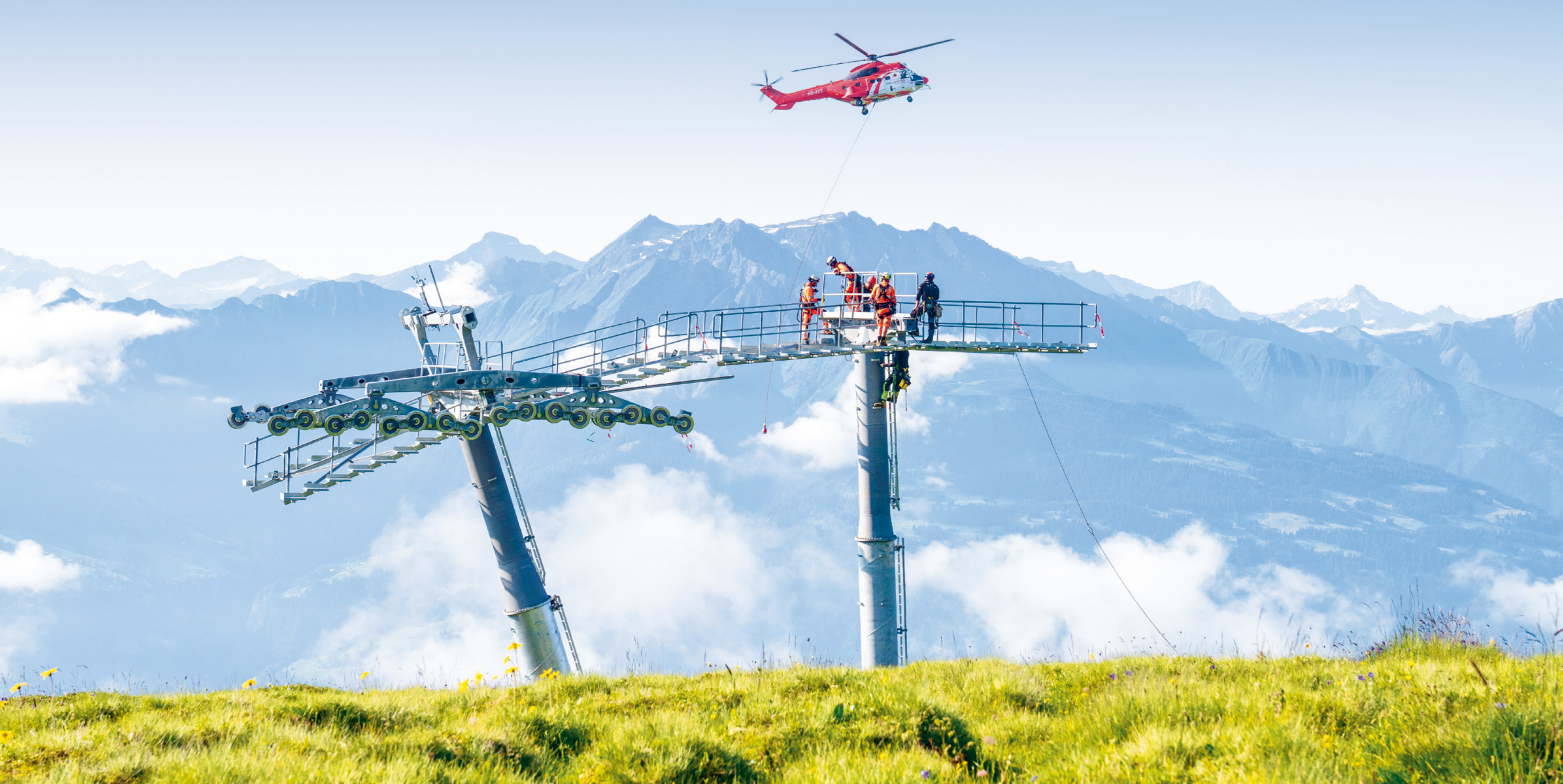
Tower Construction of Station Segnes – Nagens | FlemXpress | Films | Switzerland | Photo: © Philipp Ruggli
